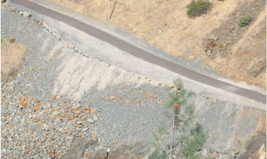
Figure 2.4. Photo of stockpiled gravel/cobble left on the parking area and hillside after the 2007 pilot injection.
