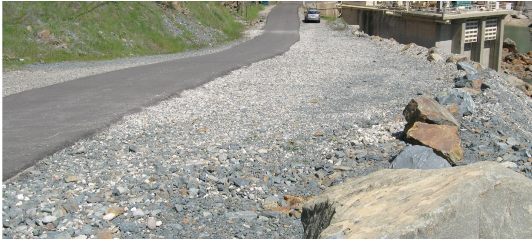
Figure 7. Residual gravel left on the parking lot surface, between boulders, and spilled over the side.
