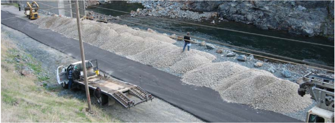
Figure 2.2. 500 short tons of gravel/cobble prior to injection into the Narrows II pool.
