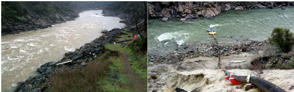
Figure 4. December 20, 2010 flow of ~14,000 cfs on the falling limb of the first flood peak that caused an injection hiatus (left); January 10, 2011 gravel injection at ~3,000 cfs using rafts to get the mixture to east bank (right). The rafts are held in place by a tether attached to a cross-channel, overhead cable. In the foreground the step descent of the sluice pipe down the hillside is shown.
