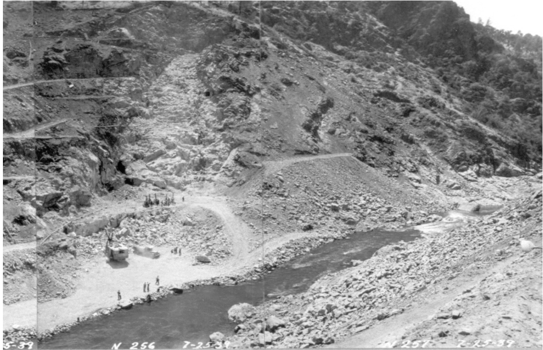
Figure 21. A steam shovel, dump truck, and five wagon drills razed the weathered canyon hillsides on July 25 th 1939 at the EDR. Large quantities of rock were stockpiled to support construction roads along channel margins and were later transported during high flow events (Courtesy: USACE, 2006).
